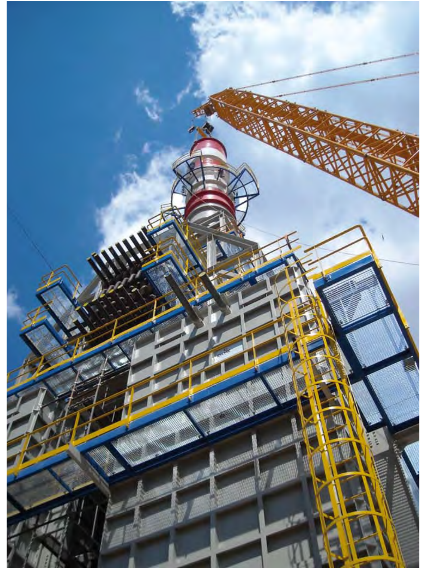
PROJECT LOCATION CLIENT / END USER Unit CDUIII 3H01 A/B Fired Heater replacement Elefsina refinery Hellenic Petroleum s.a.
