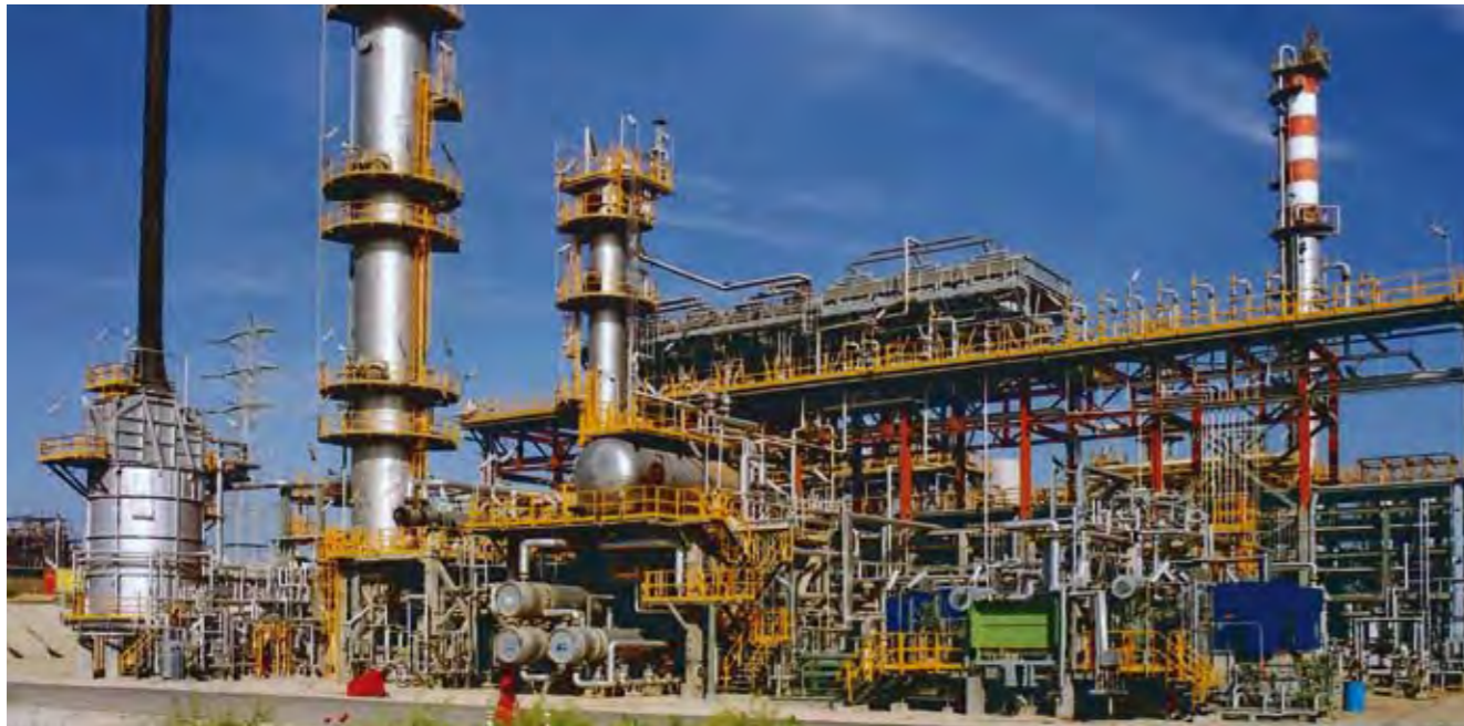
PROJECT LOCATION CLIENT / END USER Erection and electromechanical works of ULSADO unit Thessaloniki refinery Hellenic Petroleum s.a.
